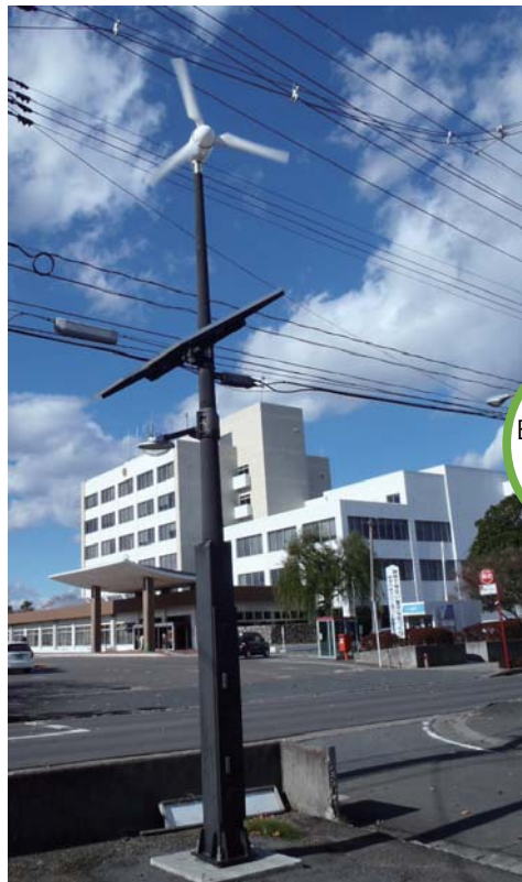
In front of City office of Natori-city, Miyagi-pref. Installation in May 2011
